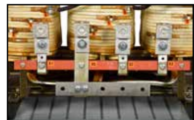
Expanded neutral bar for multiple customer connections
