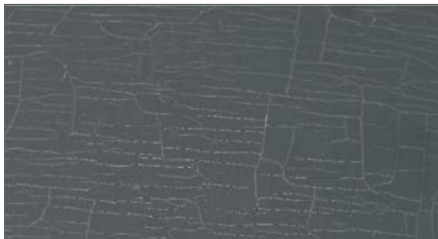
The joint has been damaged throughout by UV-radiation.
