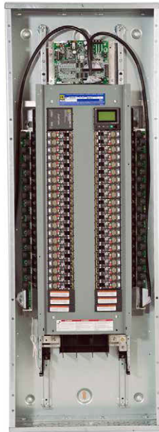
Powerlink Energy Management (EM) Lighting Control System
