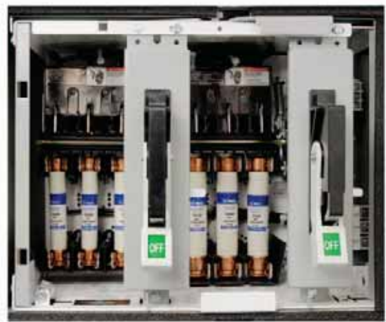
Example of Dual Feeder Disconnect Switch (DFDS)
