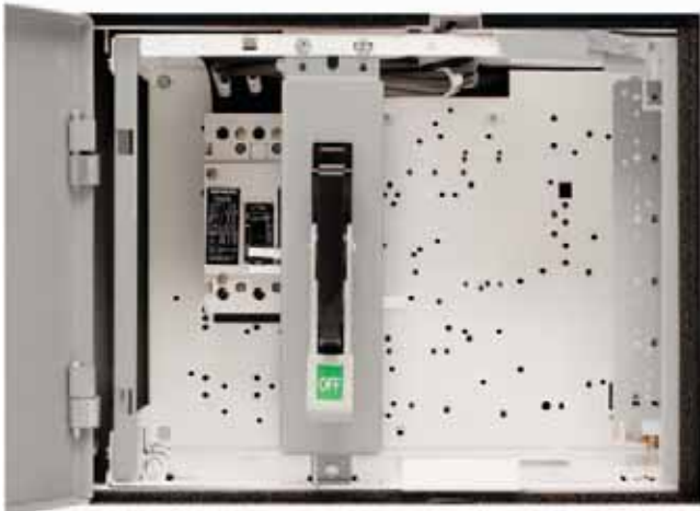
Example of Feeder Circuit Breaker (FCB)
