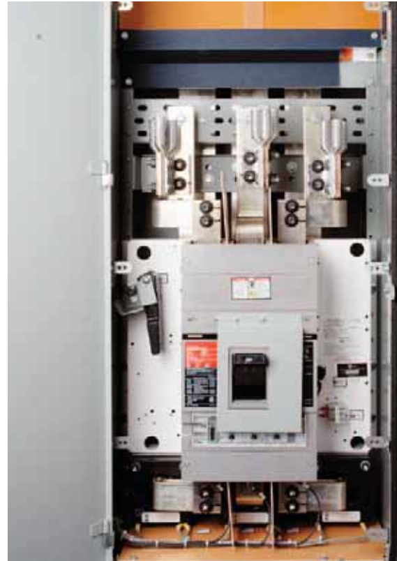
Main Circuit Breaker (MCB) Top Feed
