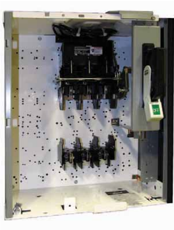
Example of 100A Disconnect Switch
