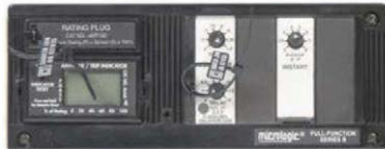
Electronic Trip Unit with Seals Installed to Restrict Access
