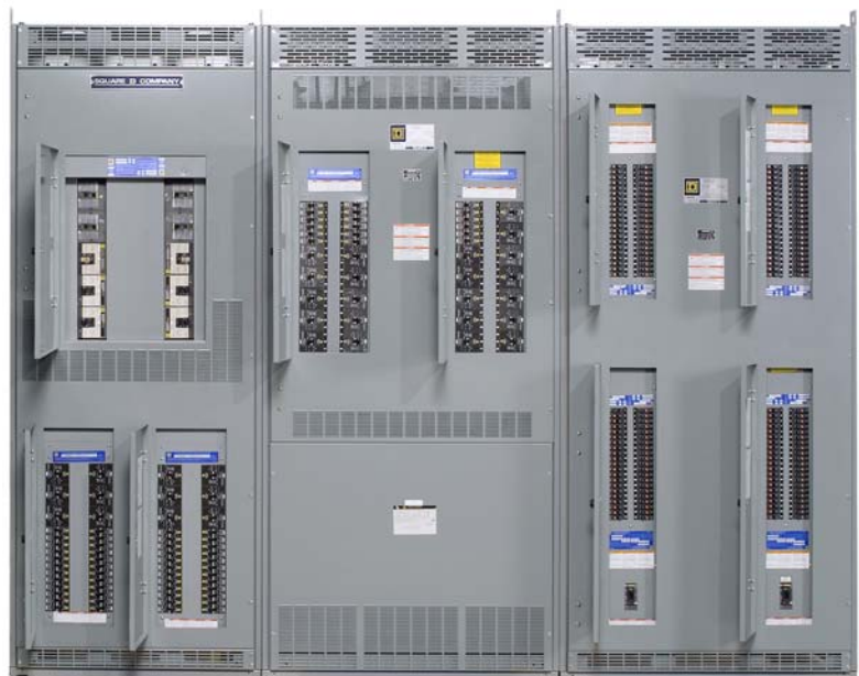
Figure 1: Integrated Power Center 2 (IPC2™)
